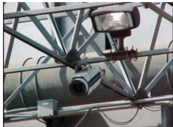
Video camera mounted to overhead gantry
