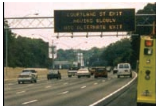
Variable Message Sign (VMS)
